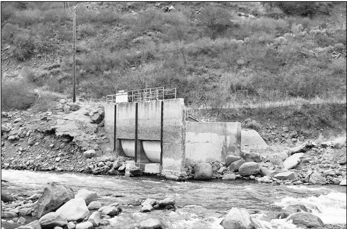
View of the project construction area looking west toward the old intake structure.
