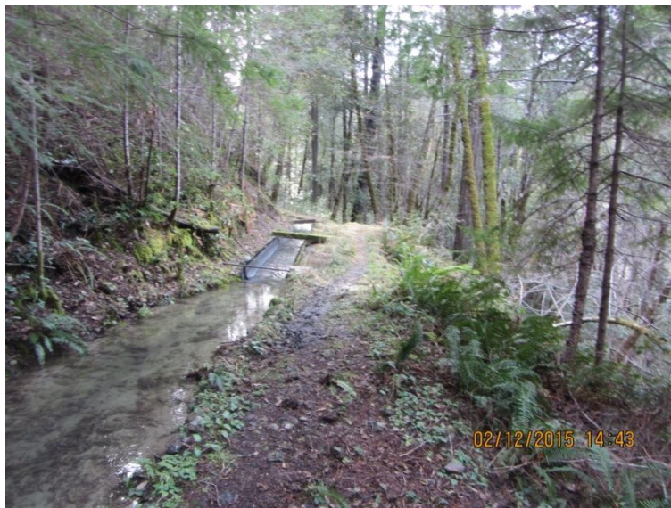
Image 12- shows Point 6, where the diversion channel is full, leaving no freeboard should it rain or the ditch receive a bank slump upstream. It appears the outboard berm may have failed in this area in the past, and at present is seeping, indicating that a portion of the berm may be saturated. Stanshaw Creek is within 200 feet; any failure here likely results in direct delivery of sediment and erosional debris. The flume section visible in the photo appears to have been installed to remedy previous ditch failures and/or to prevent future failures.
