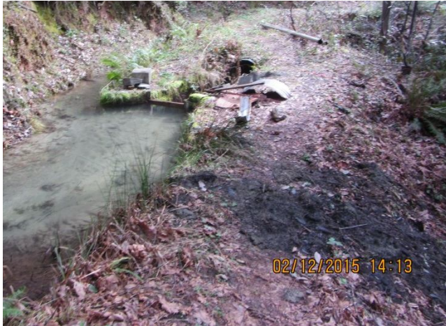
Image 10- at Point 4, shows a closer look at the seepage in the berm; note the muddy soils in the foreground. (Photo 8441 cropped)
