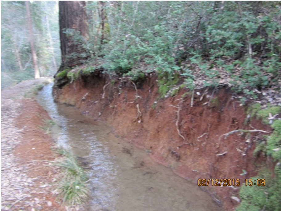
Image 23- Point 16, another cut bank that has a high risk of failure. Note the steep, near vertical slope of this cut bank, which indicates that the bank is still likely to erode. The roots hanging out of the cut bank are indicators of the erosion that has occurred. Most cut banks are originally constructed in a planar form with no visible roots protruding. Over time the cut bank erodes, exposing the roots, and leaving an indicator as to the amount of soil that has eroded or slumped. (Photo 8525)
