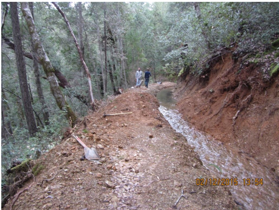
Image 24- Point 17 shows a segment of channel with an active cut bank slump and evidence of recent repairs to the outboard berm.
