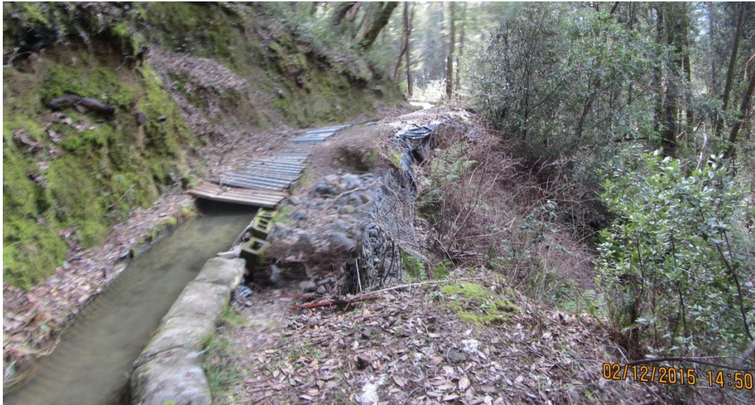
Image 15- shows Point 9, a significant failure point, likely caused by a cut bank slump filling the diversion channel and diverting the stream flow. Note the cut bank slump above and the erosion void downslope. This failure likely accelerated erosion on lower slopes and into the nearby streams. (Photo 8490 and 8491 composite)
