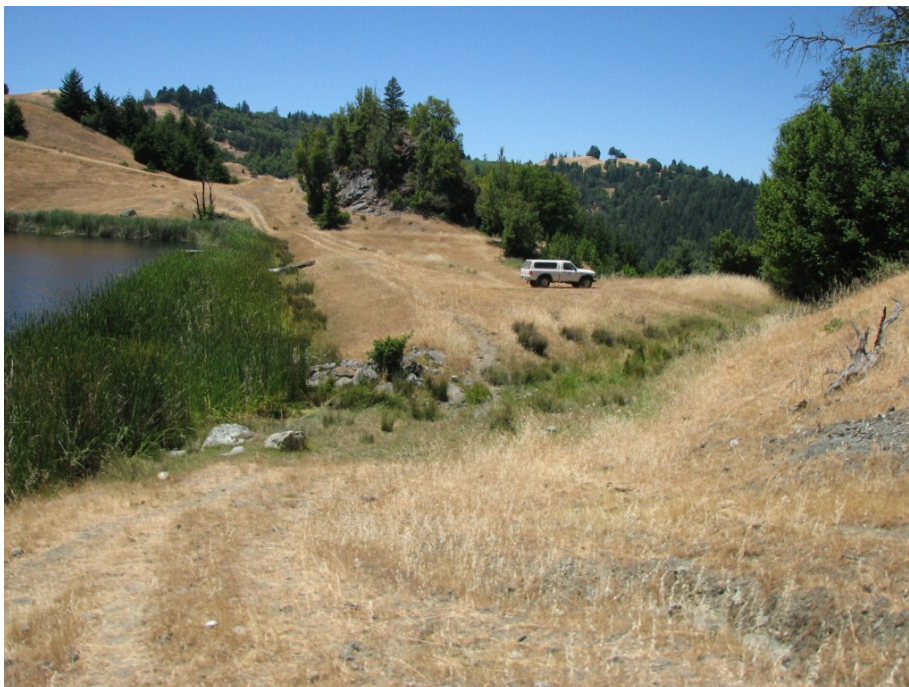
The right spillway entrance, control section and upper channel as viewed from the right abutment. Having two independent spillways adds spillway capacity and provides redundancy in the event one of the two becomes impaired.
