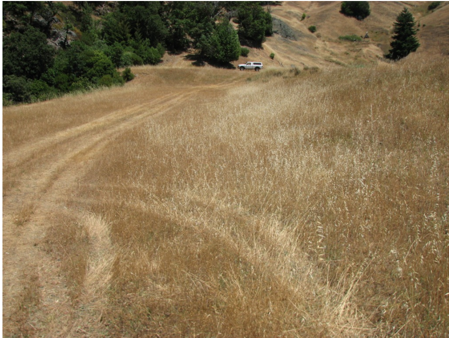
The roughly 40-foot wide downstream bench below the crest. The bench adds considerable additional width, and presumably strength, to the embankment.
