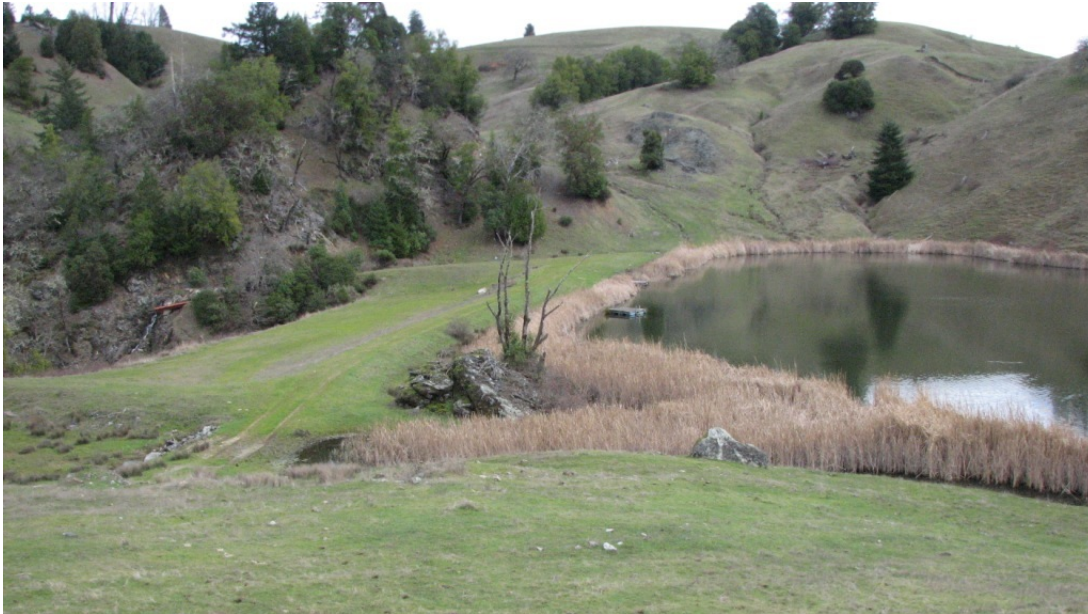
The embankment as viewed from the left abutment. Note the tule along the waterline, and the left spillway entrance channel in the bottom center of the photograph.
