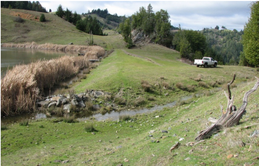
The crest and right spillway as viewed from the right abutment. Flow is about 6 inches deep in the center of the vee-shaped spillway channel.
