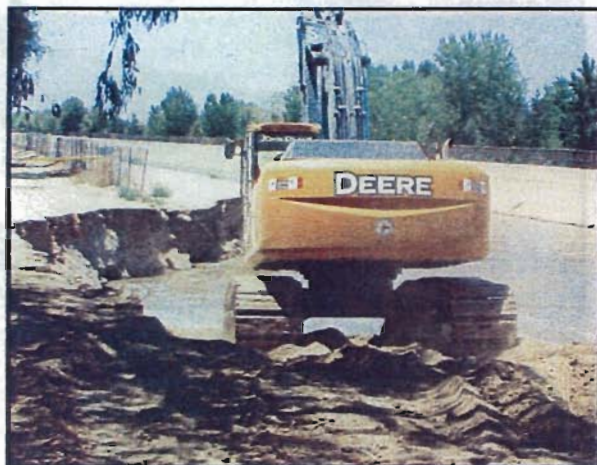
Lower Carrier Canal Washout, June 2, 2008
