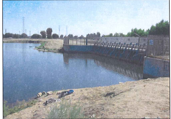
Photo h: Looking south across ponded Kern River at Riverview Park toward main gate on mainstem Kern River (near ground) and gate for Carrier Canal (in distance).
