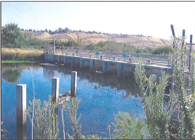
Photo c: Kern River at entrance to Beardsley Canal. Gates pond river water to facilitate diversion to Beardsley Canal.
