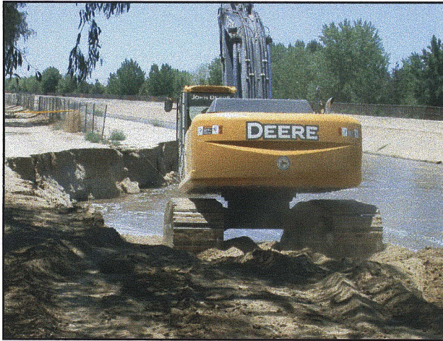
Lower Carrier Canal Washout, June 2, 2008
