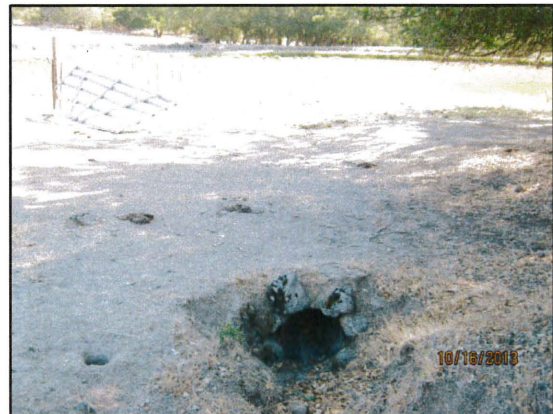
Figure 57: Third defined channel is directed through a culvert under the access road as seen looking northeast towards the reservoir.
