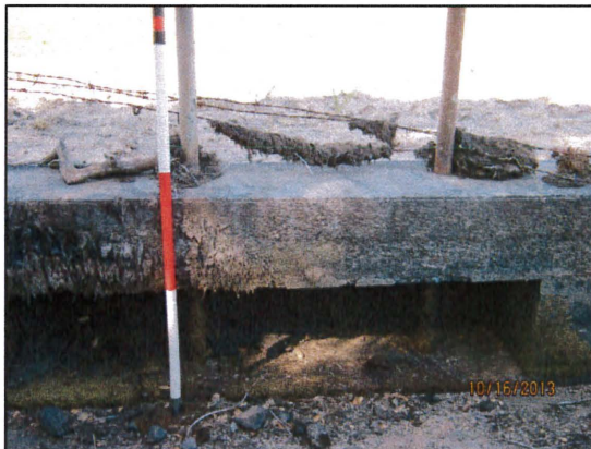
Figure 48: Screened holes in the cement wall now covered by sediment. Dried reservoir surface cover tangled in the wires above the cement wall.
