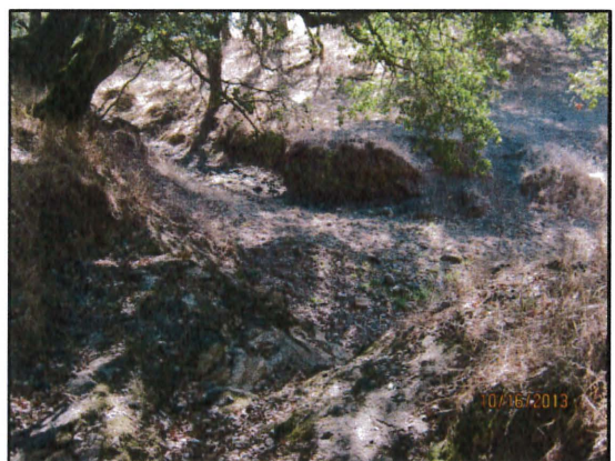
Figure 63: Defined spillway channel at the Unnamed Stream. Unnamed Stream below the dam flows southeast to the property line.
