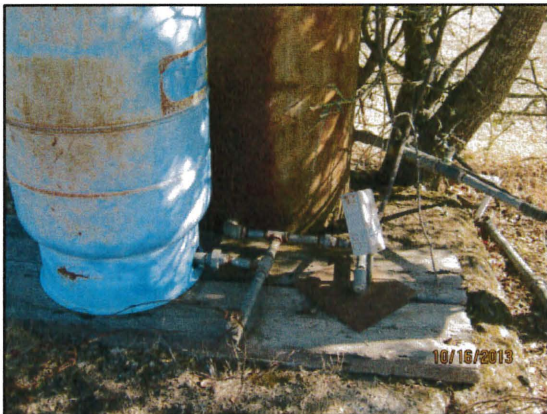
Figure 54: Water well platform and connections.
