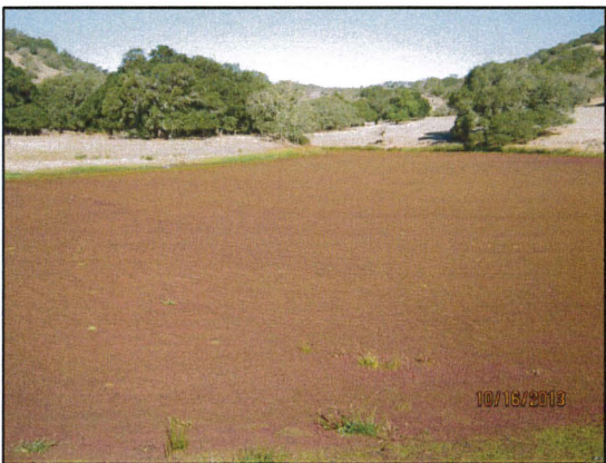
Figure 38: From the spillway looking northwest across the reservoir. It appears the grassy vegetation in the foreground is growing on top of the reservoir surface cover.
