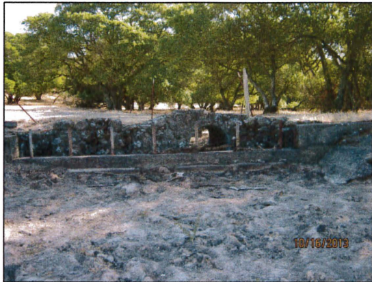
Figure 46: Spillway at the northern end of the earthen dam. Cement wall in front of the spillway pipe is backfilled with sediment.
