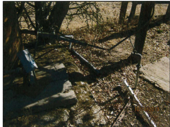
Figure 55: Water well piping.
