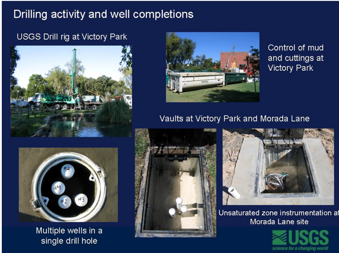
Figure 7-26 Installation of Monitoring Wells in Victory Park, Stockton. Note examples of multiple cluster well types.
