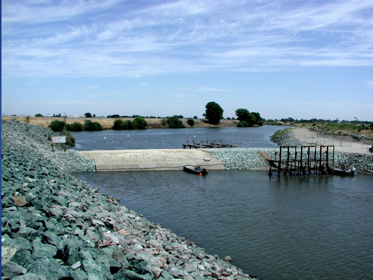
Typical rock barrier with culverts and slide gates (Head of Old River)
