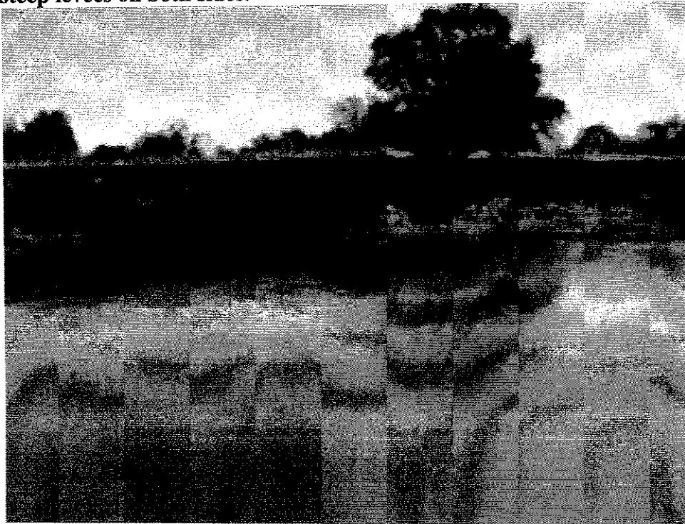
Figure 12. In some areas of the lower San Joaquin River, the steep levees have begun to erode.
