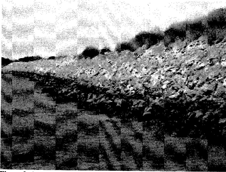
Figure 9. An example of the steep, rip-rapped banks of the lower San Joaquin River with limited or no vegetation.
