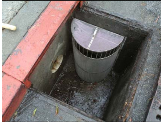
Figure 2.1. Example storm drain inlet screen utilized as a monitoring site.
