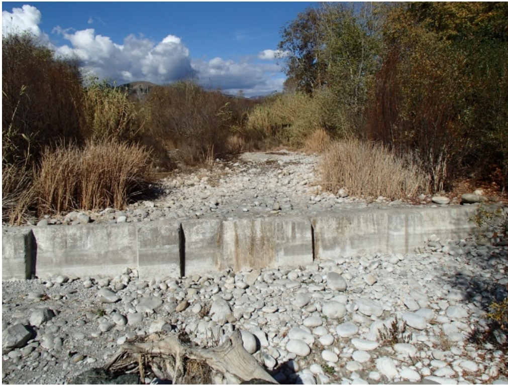
Figure 2. Dry Ventura River at the Foster Park subsurface dam and diversion on November 22, 2013. Dry conditions at Foster Park were prevalent throughout the 2013 - 2014 dry seasons.
