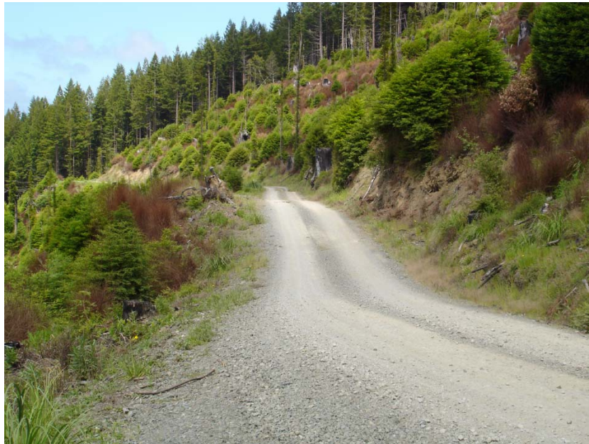
Figure 19. Example of road segment built to drain properly in wet weather. Note the two functional dips and their spacing.
