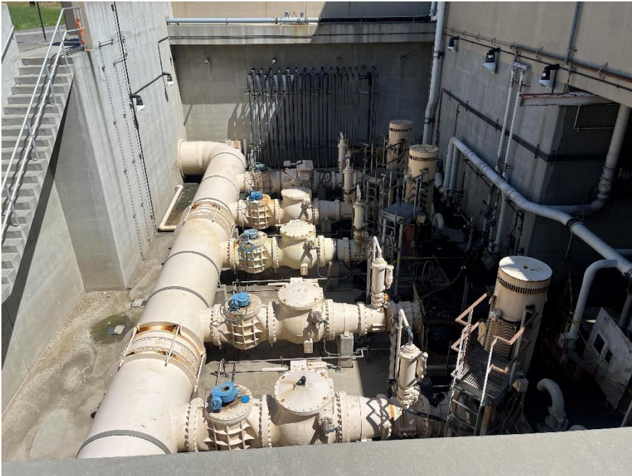
Figure 5: Influent pumps. (MC 04/03/2024)
