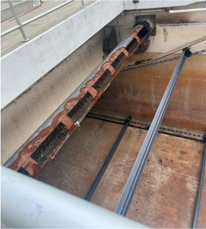
Figure 9: Skimmer trough at PST No. 5. prior to resuming service (MC 01/10/2024)
