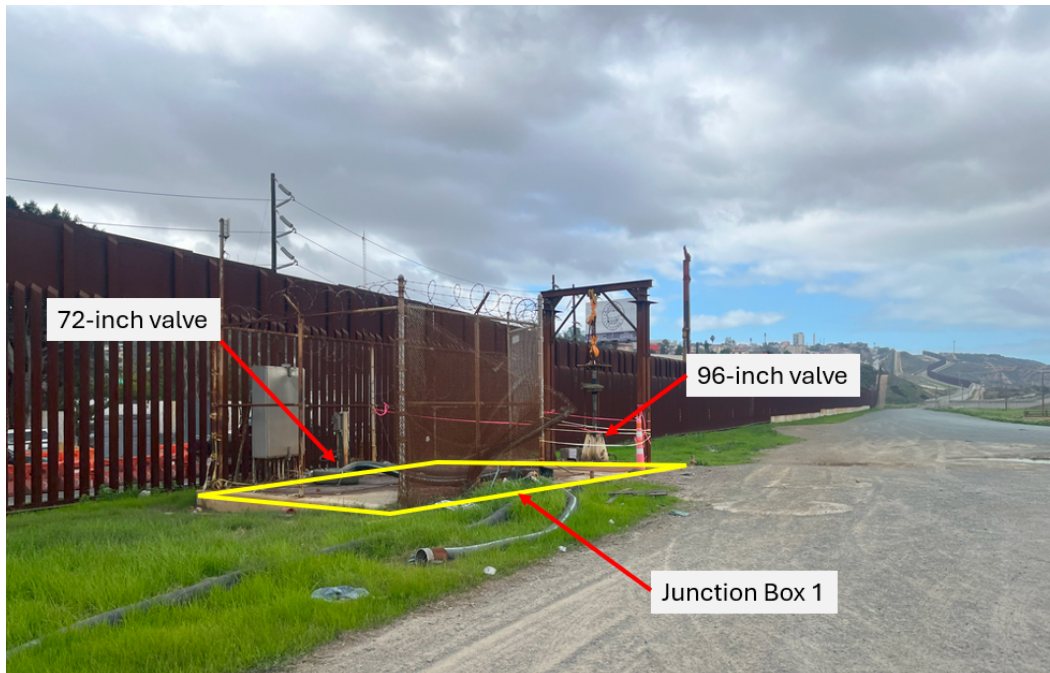
Figure 4: Junction Box 1. (MC 01/10/2024)
