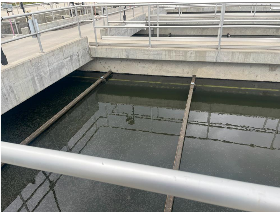
Figure 12: Secondary settling tank. (MC 01/10/2024)
