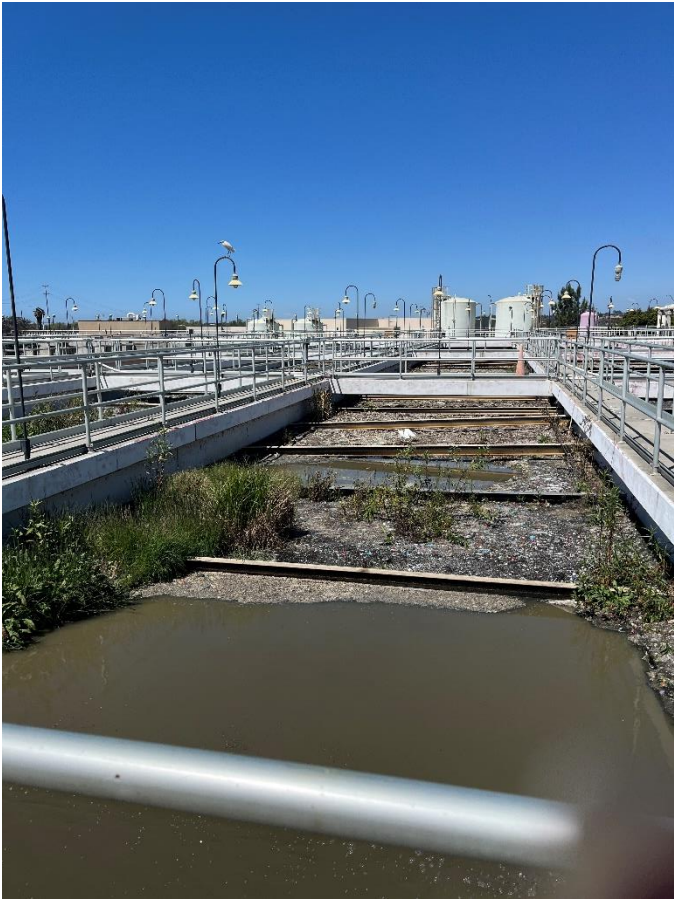
Figure 10: One of four inoperable PSTs. (MC 04/02/2024)
