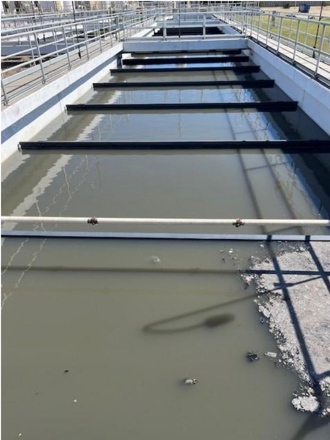
Figure 8: Rehabilitated PST No. 5. in service (USIBWC 04/17/2024)
