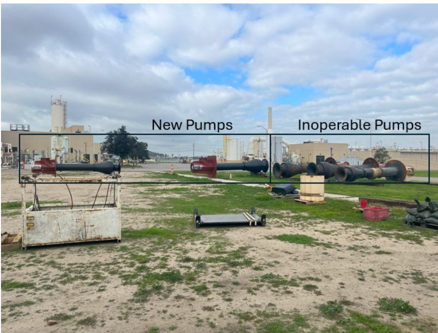
Figure 6: Two new influent pumps on the left. Three inoperable influent pumps on the right that have been removed for replacement. (MC 01/10/2024)
