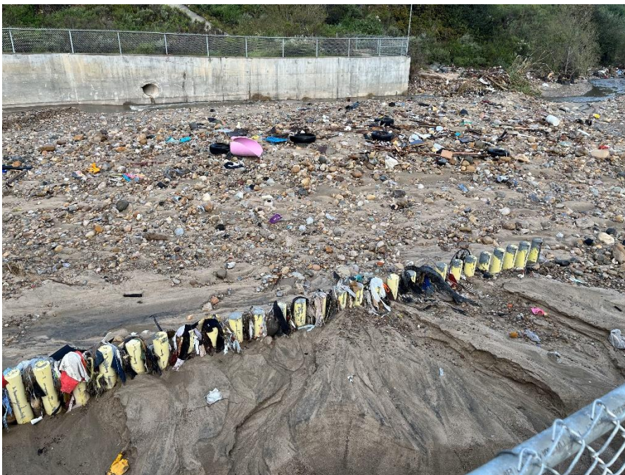
Figure 2: Trash and sediment at Smuggler's Gulch Canyon Collector. Bollards are approximately five feet in height. (Veolia 04/01/2024)
