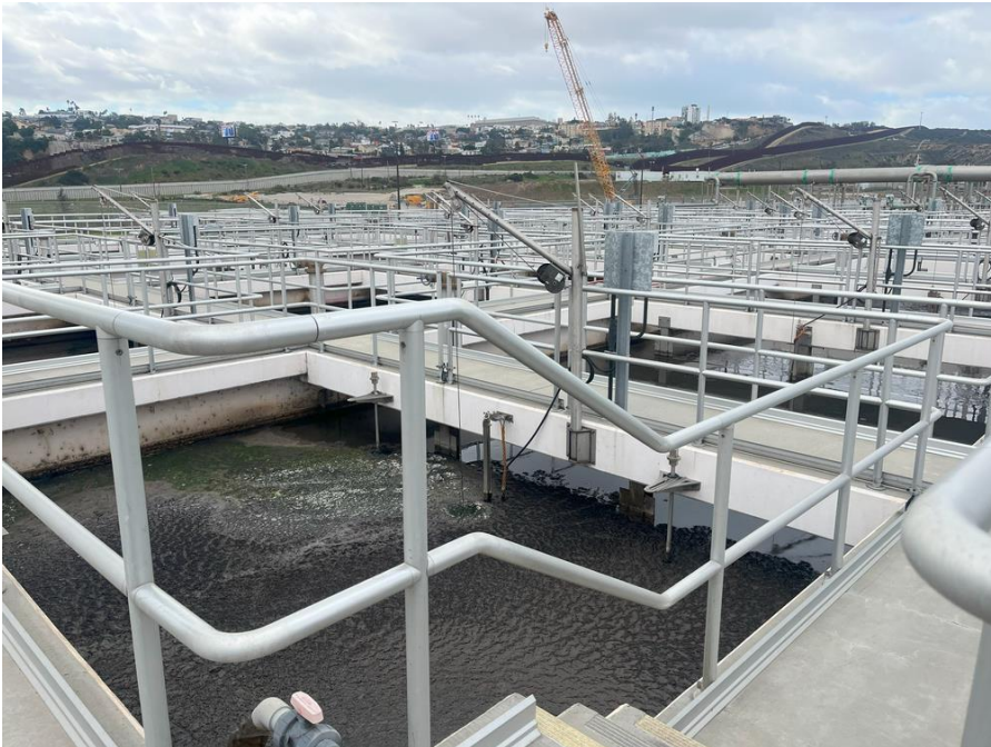
Figure 11: A photo of a secondary mixing tank.
