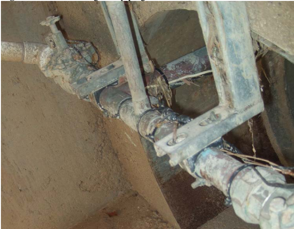
Figure 2-4. Private irrigation piping in storm drain
