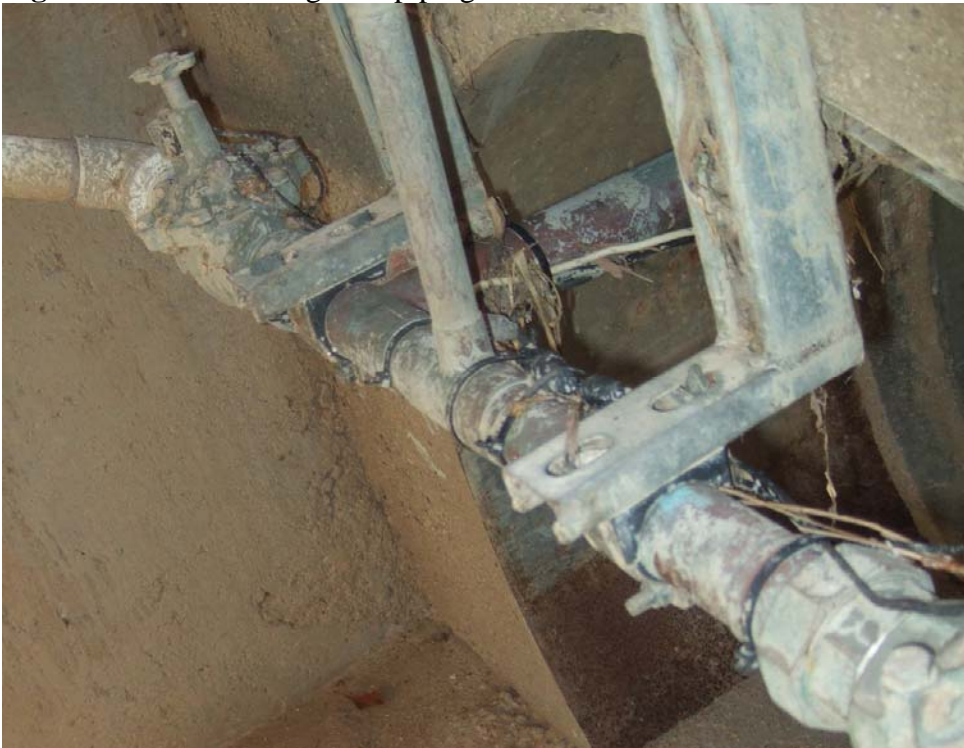
Figure 2-4. Private irrigation piping in storm drain
